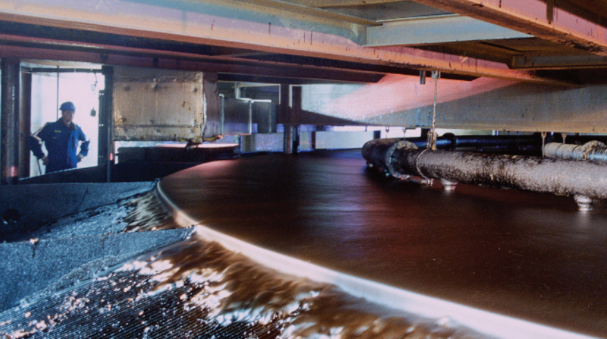
Suncor's primary extraction plant, near Fort McMurray, Alberta, separates raw bitumen from sand in this giant separation cell. (Photo courtesy of Suncor Energy Inc.)
